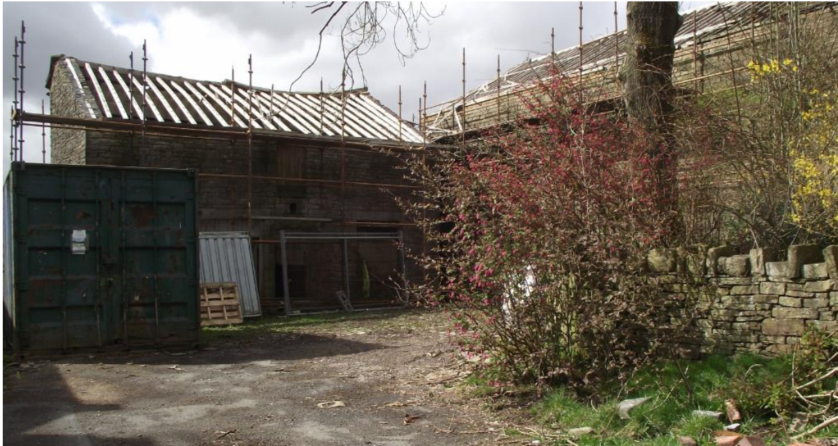
Photograph taken 2 nd April 2020 – showing unauthorised works to the roof.
